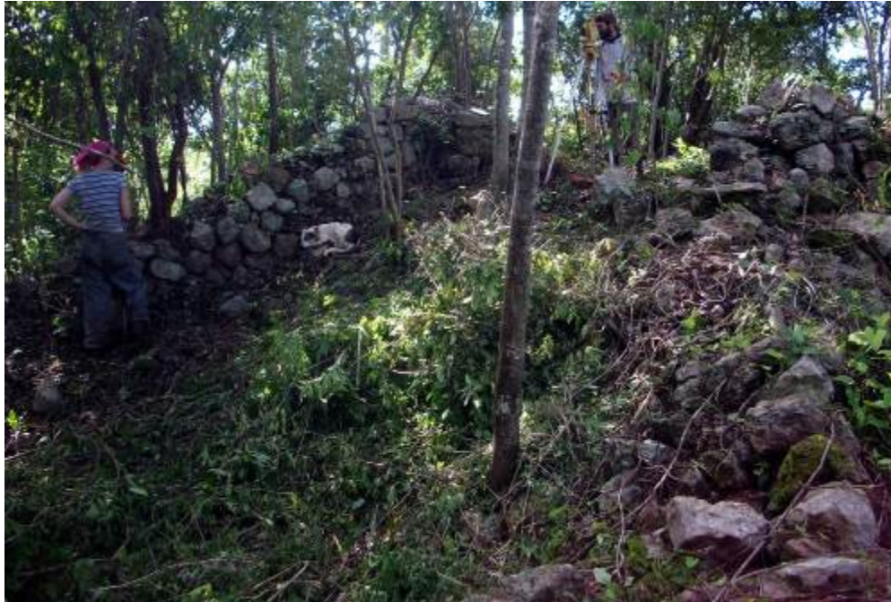
Figure 23. Difference in the Ground Level between the SE Bastion and Western Side of the Fortalice of Yo'okop
